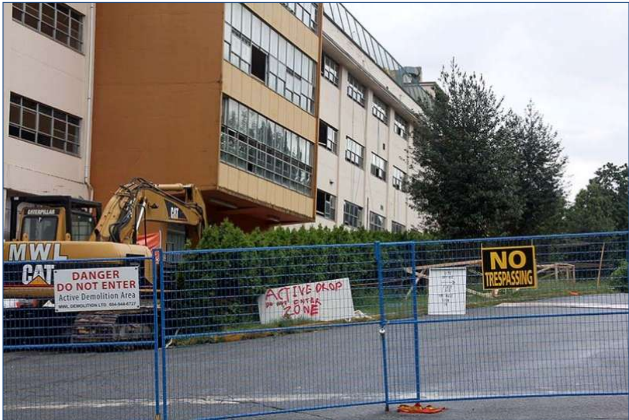
Sadly, demolition of the Valleyview building on the Riverview Hospital grounds has already started. Bruce Brandhorst photo.
